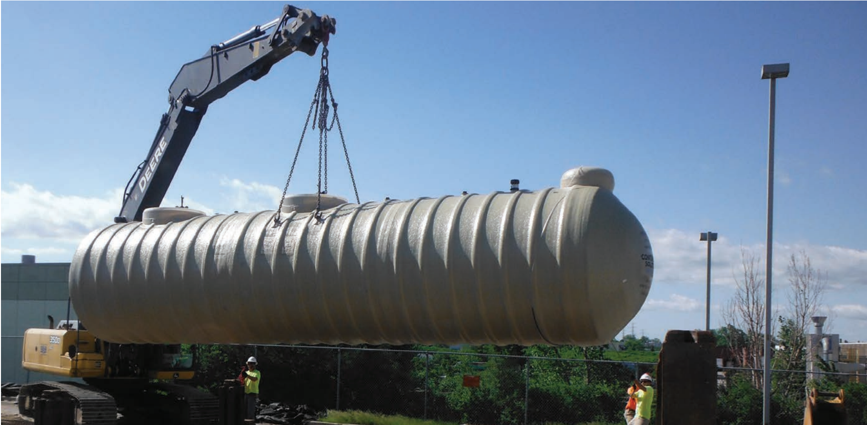
USPS storage tank
