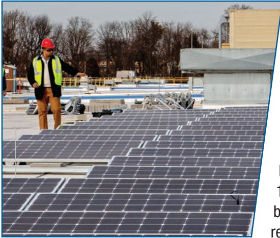
Solar panels on USPS facility
