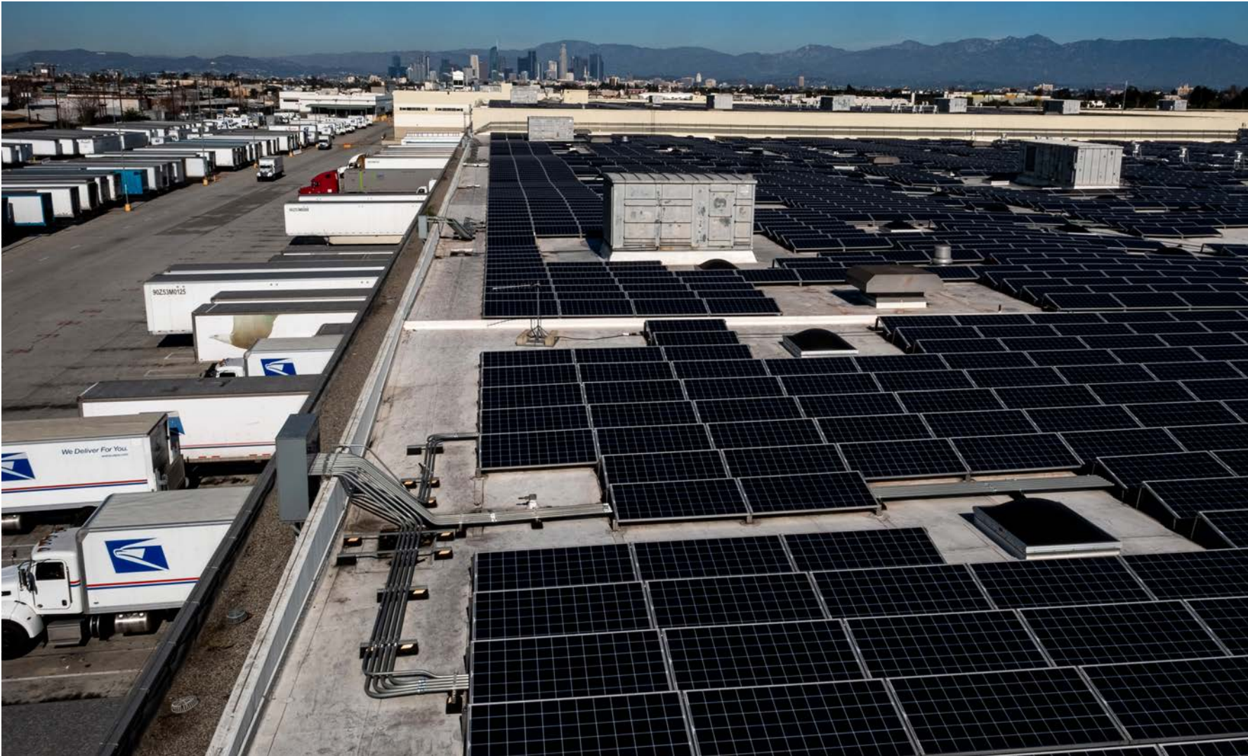
Solar panels in Los Angeles
